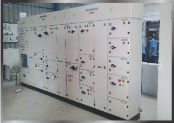
MCC CONTROL PANEL
