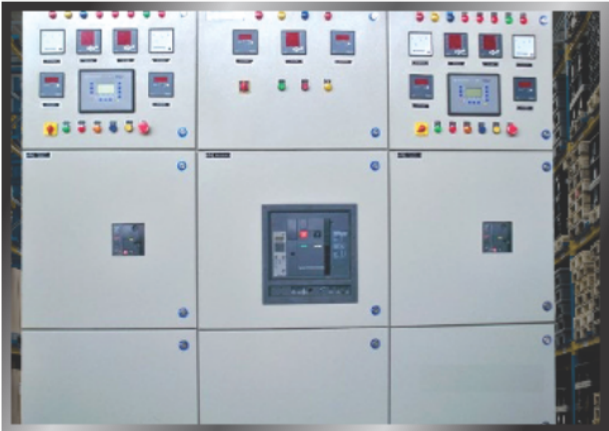
DG SYNCHRONIZATION PANEL
